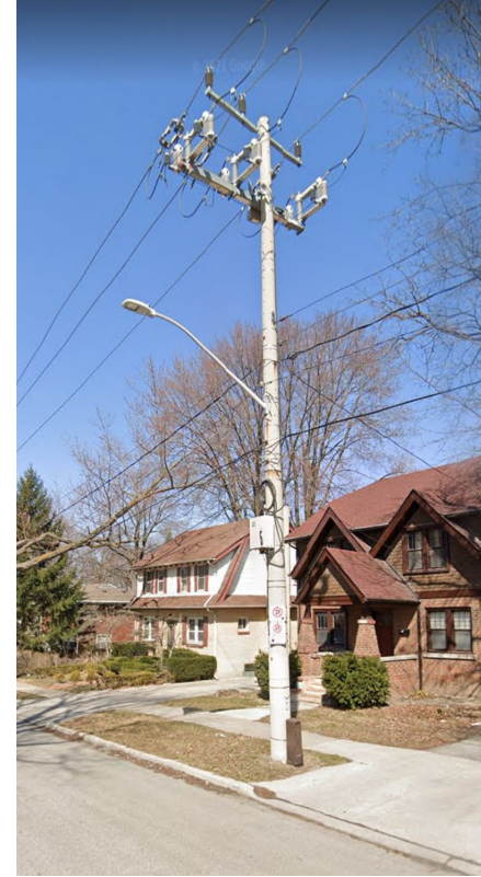
34.5 kV, 600 A Motorized Switch
