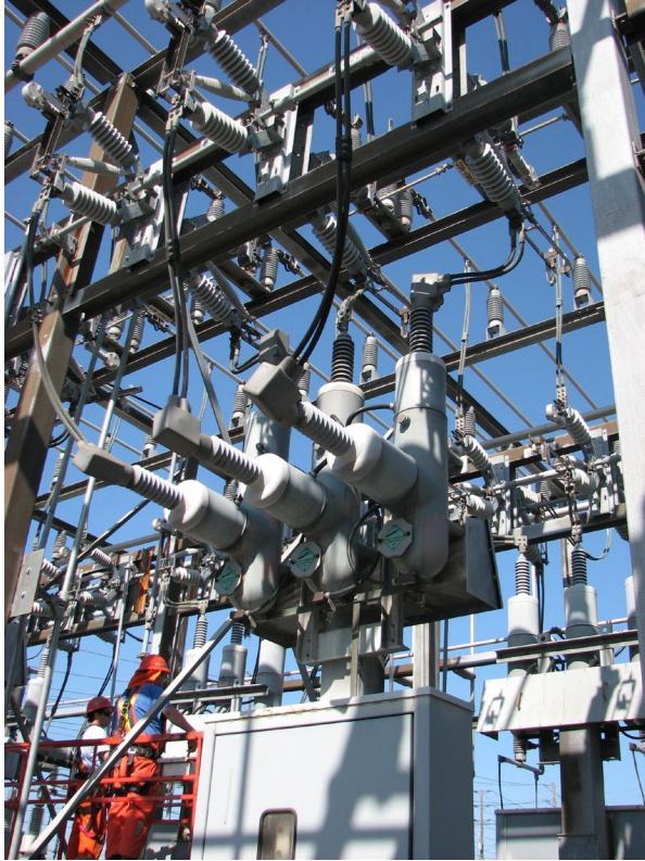
34.5 kV, 1200 A Feeder Breaker
