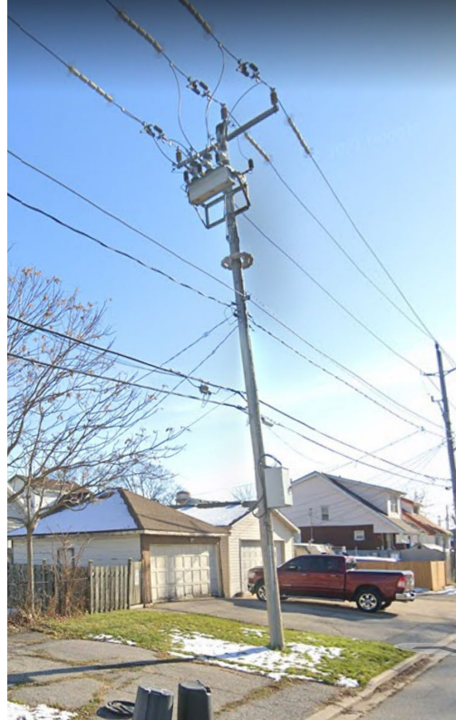
34.5 kV , 630 A Recloser
