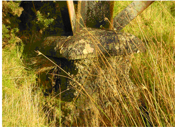
Figure 7: Deterioration of Overhead Line Steel Tower Foundations
