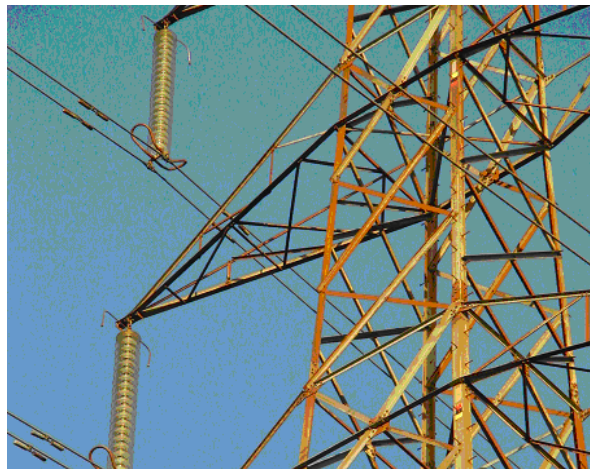
Figure 6: Lattice Overhead Line Steel Tower Corrosion
