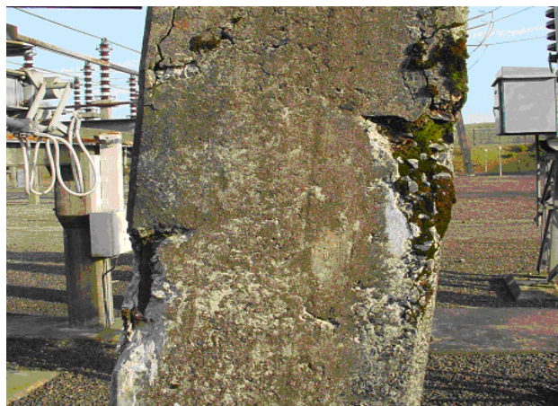
Figure 9: Degradation of Civil Structures within a Switch Yard
