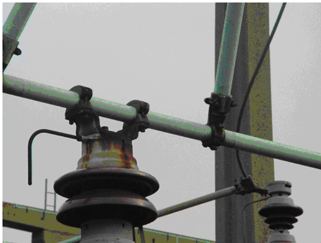
Figure 12: Busbar Clamp Corrosion
