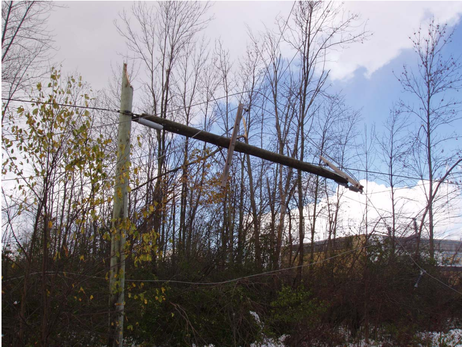
New poles sheared.
