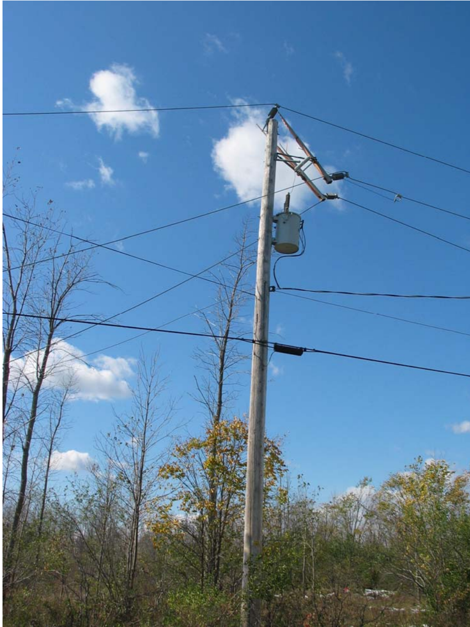
Cross arms broken from loading of snow, wind and trees.
