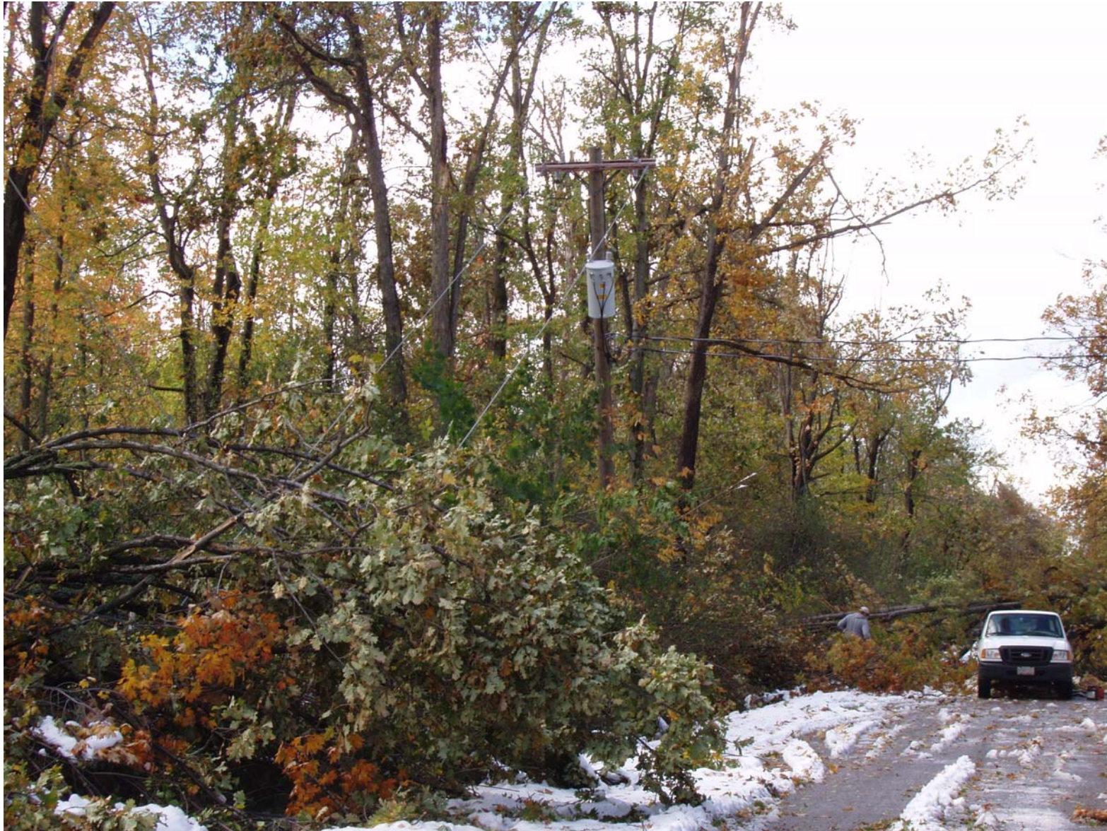
Newly constructed pole lines broken because of high tensile strength of ACSR.
