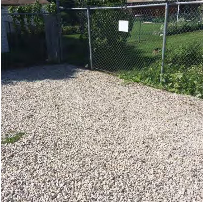
-gap below fence fabric
